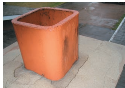
Damaged crown and eroded mortar joints should be repaired before relining.
