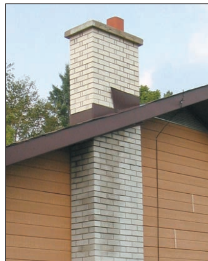
Stains like these are caused by condensation of moisture and creosote from cool flue gases.
